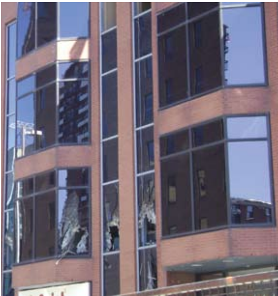
Co-operative House, shortly after the fire that damaged CCA's offices.
